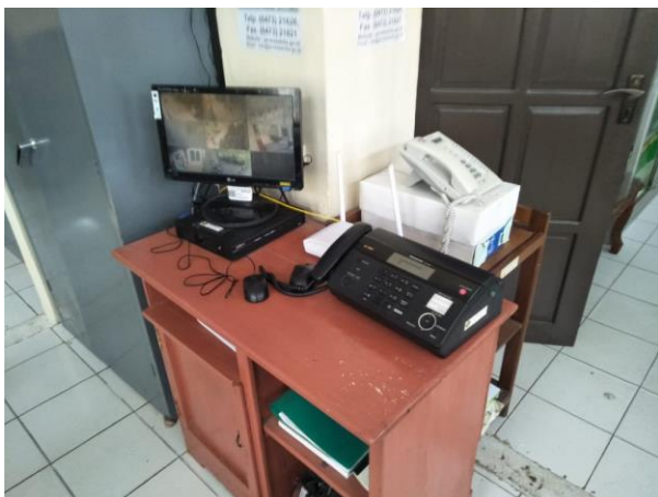
Ruang control CCTV
